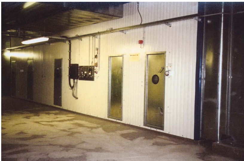
Supply Air Unit
